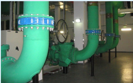
Burj Khalifa District Cooling DCP3 (Dubai)
