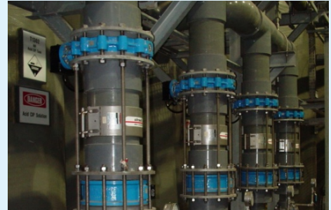
Ulu Pandan NeWater plant (Singapore)
