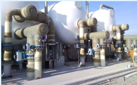
Delta de la Tordera Desalination Plant (Spain)
